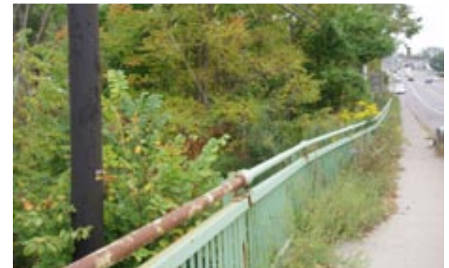
Maintenance on public and private land is lacking
